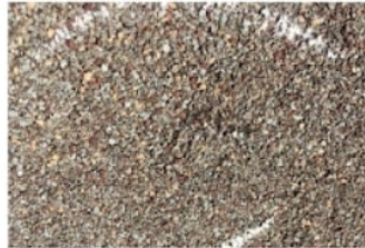
Hail Damage After Storm
