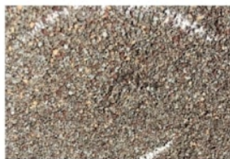
Hail Damage After Storm
